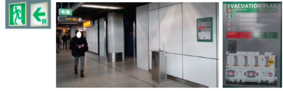
Figure 3. Evacuation guidance media and promotional signage ( PS ) at a terminal. (Left: exit sign ( ES ). Middle: evacuation plan. Right: evacuation map on the wall.).
